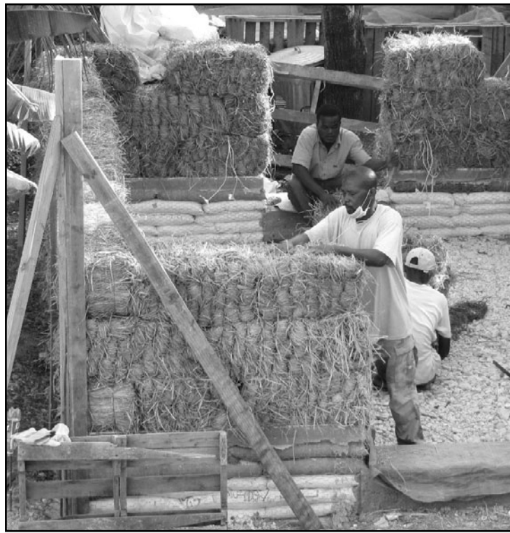
Left, Haitian workers build a straw-bale house. Below, Andy Mueller, a Charlemont resident who is the lead builder in the "Ti Kay Pay" project, is hoping to teach Haitians how to build the inexpensive, energy-efficient shelters that could help reduce some of the homelessness, food-scarcity and even the building rubble left after last year's earthquake.
